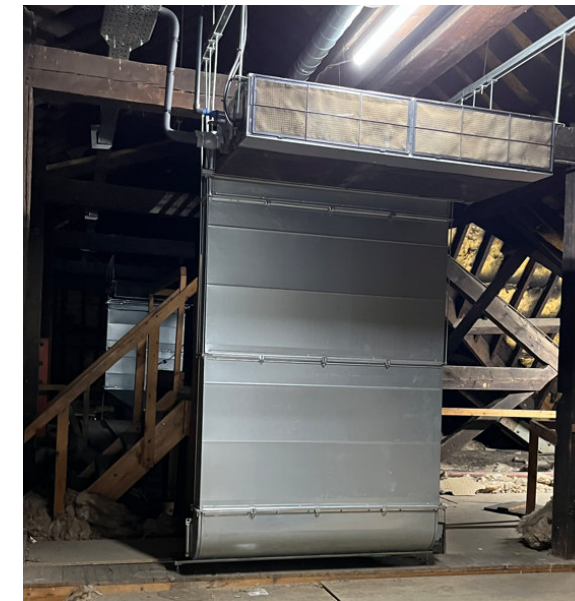
Ducted heating and cooling units to Victoria rooms within loft space, provided by fresh air by local fans. Unit over large venue/conference space.
