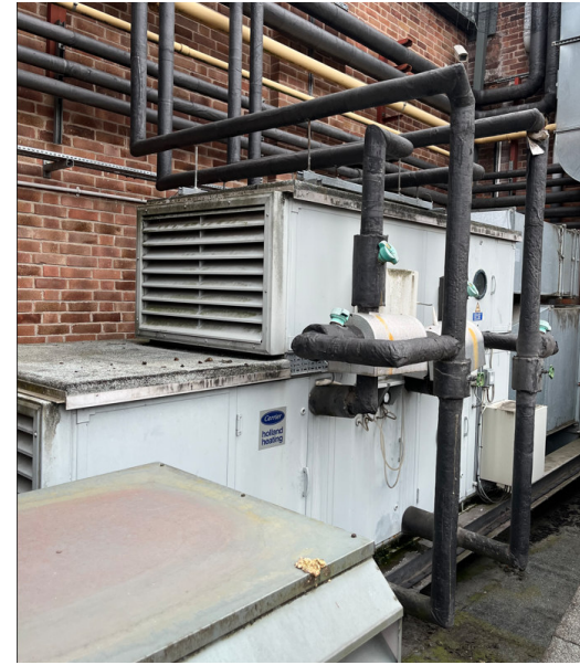
AHU03 in plant area outside mezzanine plantroom, serving kitchen.
