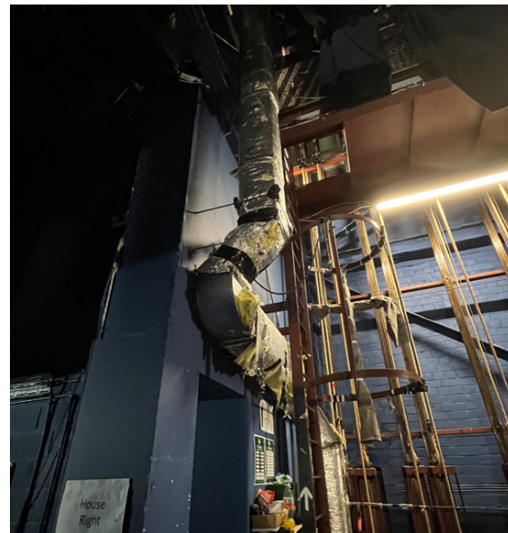
Services to backstage areas are particularly deteriorated. Ventilation distribution systems in particular are showing signs of extreme signs of aging past life expectancy. Backstage area was noticeably warm at time of visit whilst unoccupied.
