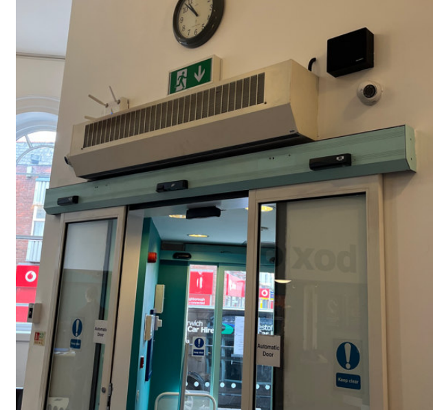
Overdoor Air Curtain to entrance draught lobby.
