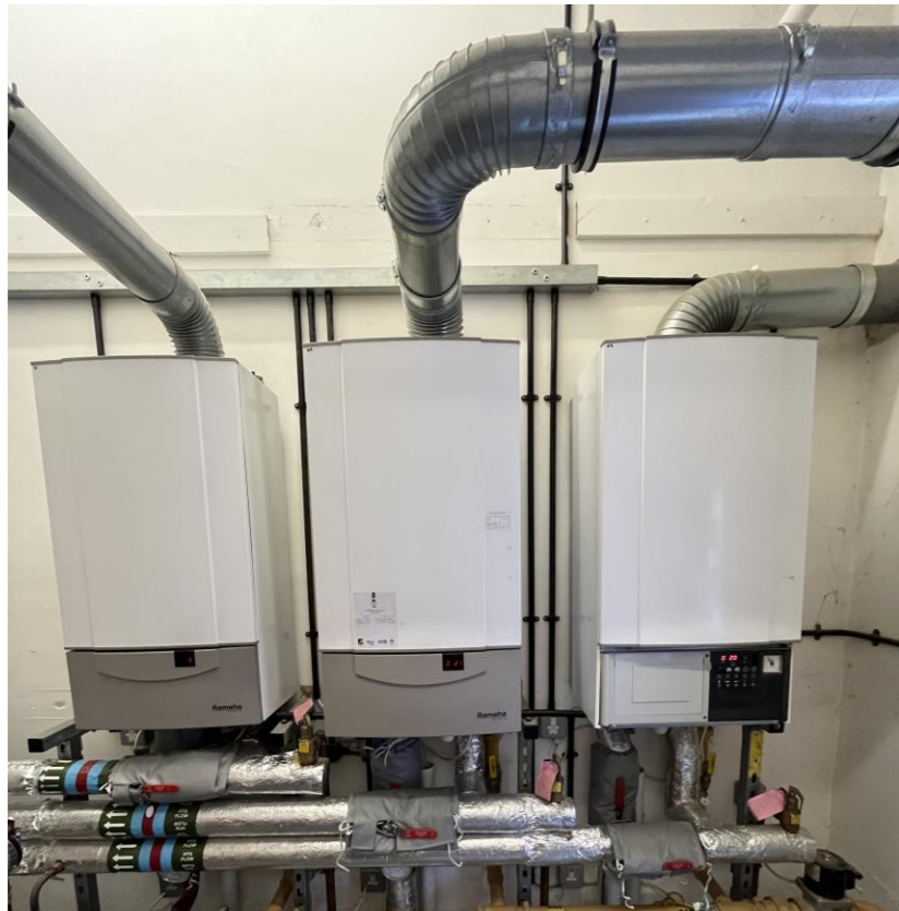
Existing Gas Fired Boilers
