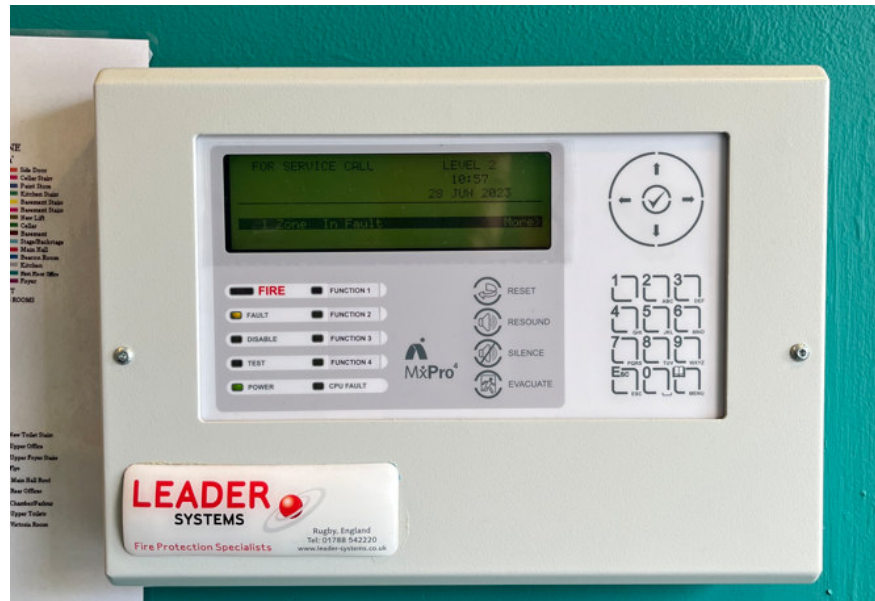
Fire Alarm panel in entrance lobby to Town Hall.
