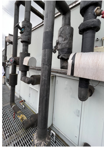
AHU01 in external plant area outside mezzanine plantroom, serving main performance hall.
