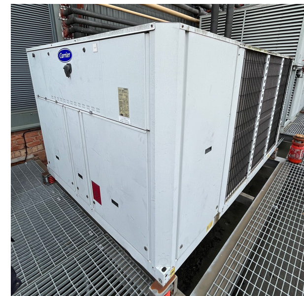
Carrier Cooler in external plant area outside mezzanine plantroom. New unit has been ordered outside of any contract works and therefore is to be replaced directly by town hall maintenance team.
