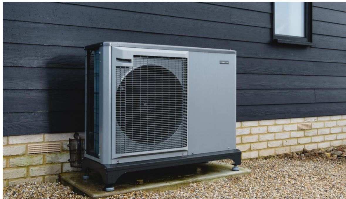
Air Source Heat Pump
