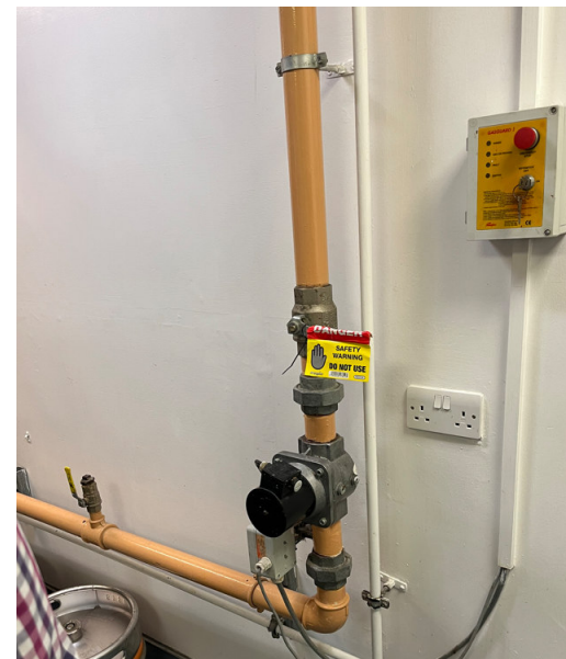
Existing kitchen gas incomers with solenoid valve and gas safety system.
