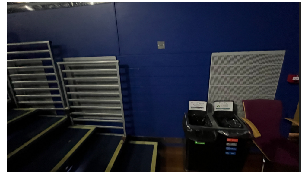
Performance hall ventilation grilled run along either side wall of the hall itself in the form of sidewall grilles providing ventilation, with heating and cooling provided by treating the incoming air. Air delivered below the bleacher seating.
