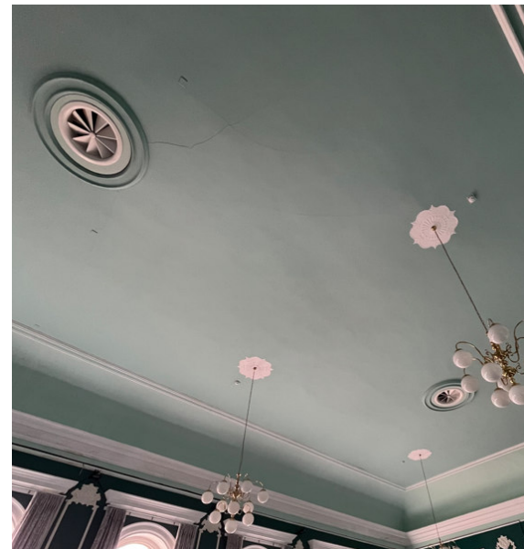
Air terminals in Victoria Room
