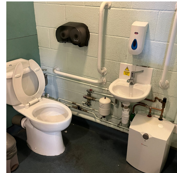
Many WC's beyond the performance areas have local electric point of use water heaters and direct electric showers, a number of which are not working and redundant – requiring replacement.
