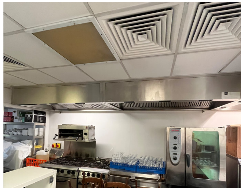
Kitchen Ventilation includes both 4 way blow grilles within ceiling and 2No. ventilation canopies over cooking equipment.
